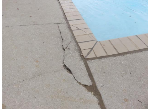
Significant pool deck cracks
