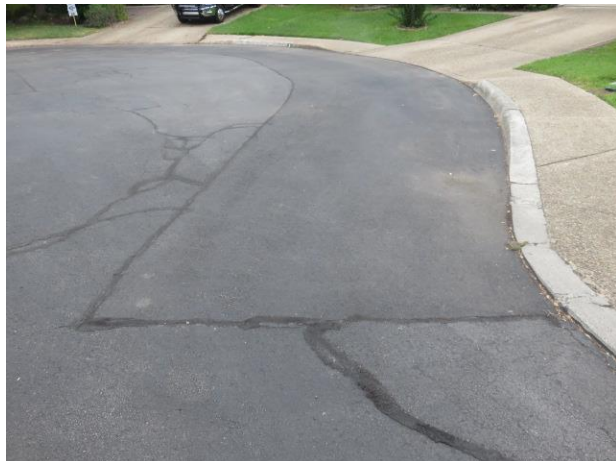
Large patch at cul-de-sac
