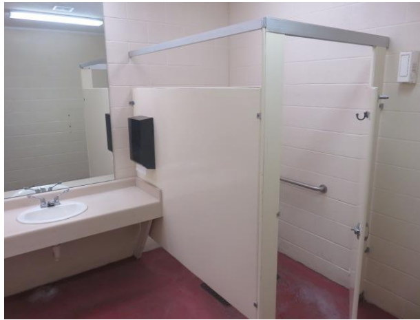
Rest room plumbing fixtures and partitions
