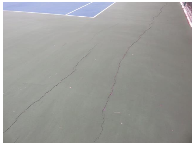
Typical cracks at tennis court edge
