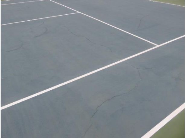
Cracks at tennis court playing surface
