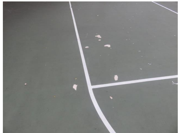
Color coat deterioration throughout basketball court
