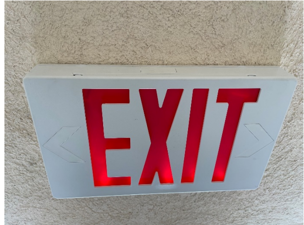
New EXIT sign.
